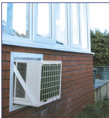
View of Debonair unit from exterior
